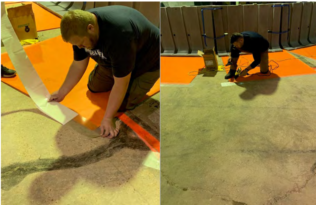
Figure 12. The orange base liner being taped to the floor and application of heat.
