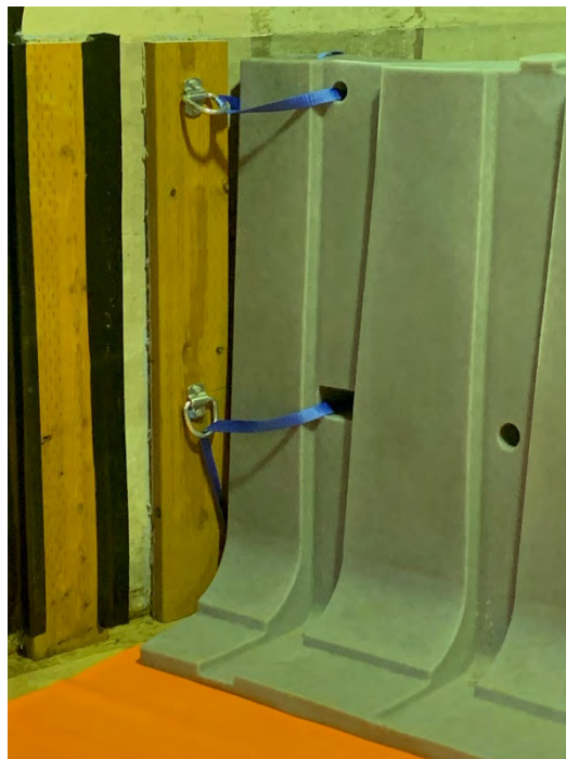
Figure 10. Placement of ratchet straps to cinch the barrier with the basin right wingwall.
